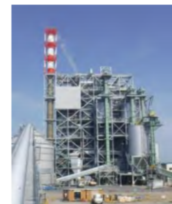
Biomass boiler at MPM Oji Eco Energy 25
